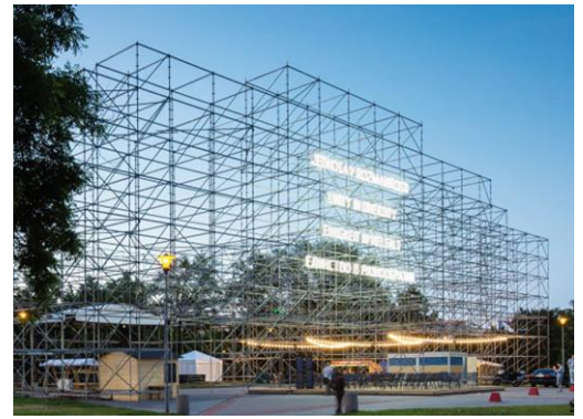
Right, the scaffolding version of the German House, erected in the same location in 2017
